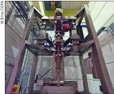
Installation of the GBAR linac in its shielding bunker.
